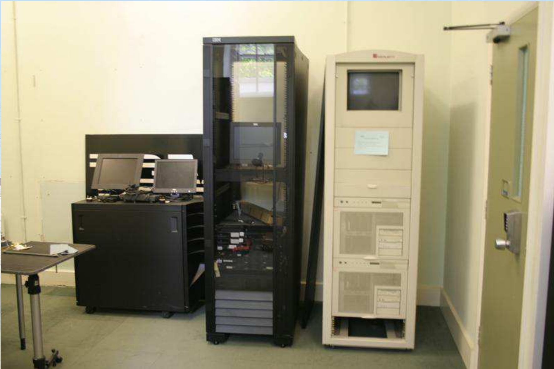
Rack, Sequent Rack
