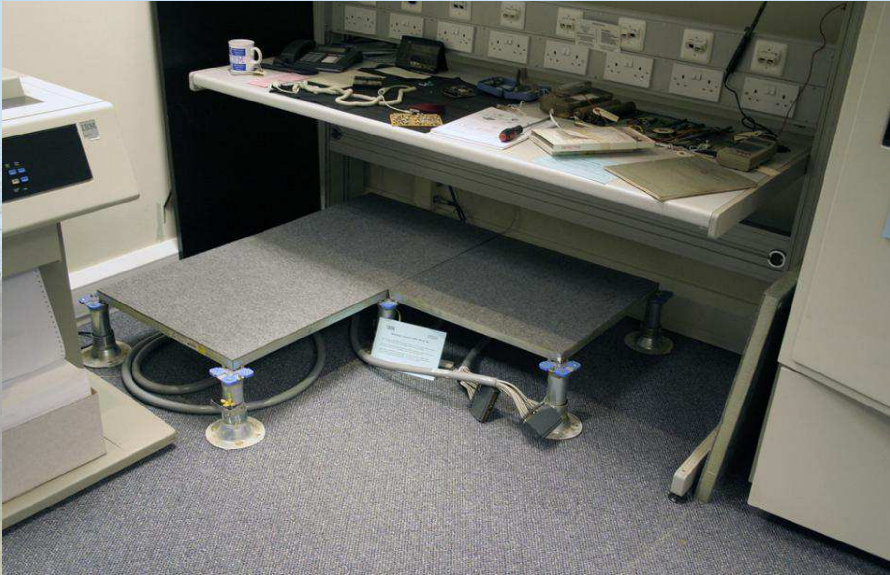
False Floor with Channel Cables
